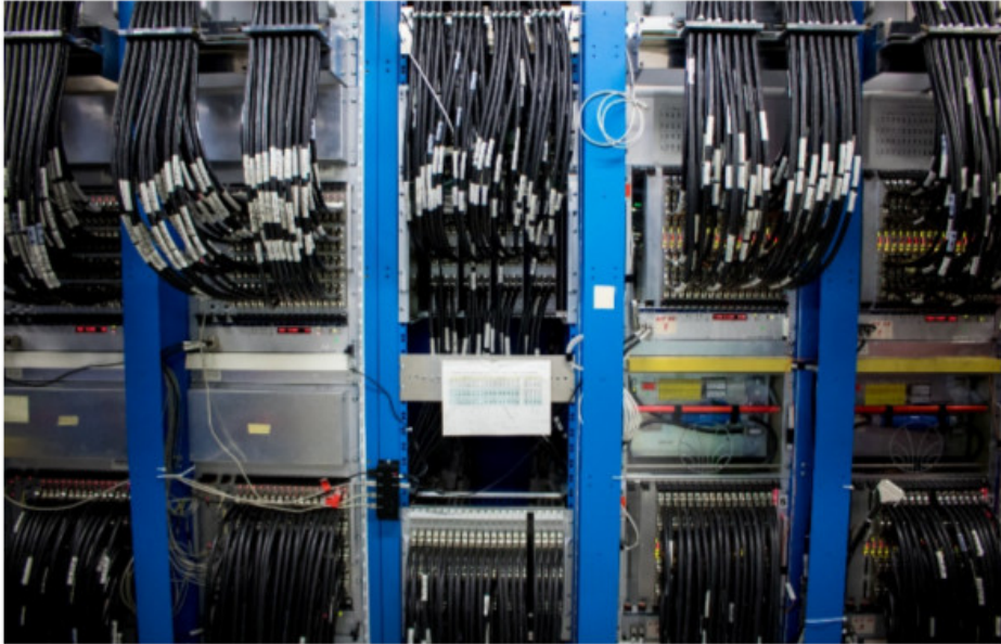
Figure 2.13: Racks of the first-level calorimeter trigger system installed close to the detector.
