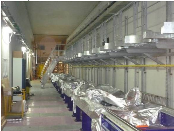
Figure 11: linac and valve boxes support in the tunnel.
