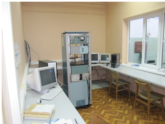
Figure 8: NESTOR facility control room.
