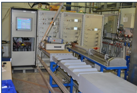
Figure 8: First cabinets of solid state amplifiers being tested at GANIL on the variable VSWR test bench.
