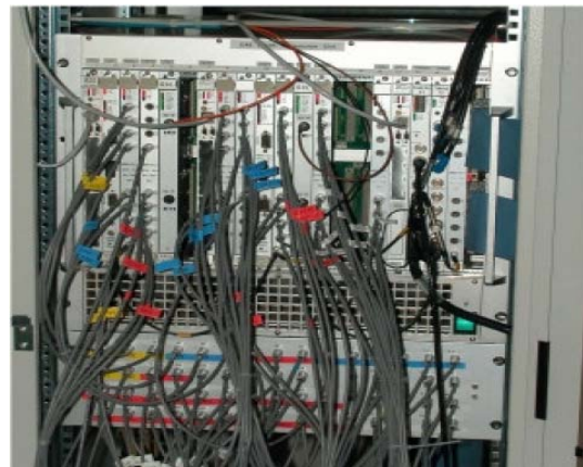
Figure 3: An image of the local control
