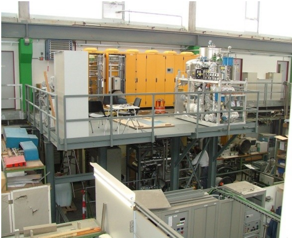
Figure 4-1 : The MITS at PSI in March 2004: The oil loop in place at the right hand corner of the platform (thermally insulated, but still uncovered), the WCL underneath, and the racks of the control system in the rear. A wooden plate covers the target reception flange in the middle of the MITS.
